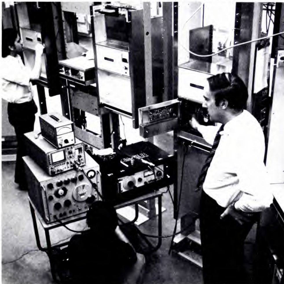
The equipment shown here in system test is part of a microwave network which extends CPB programming from Sprague, Washington to ETV stations in Pullman, Washington and Moscow, Idaho.
